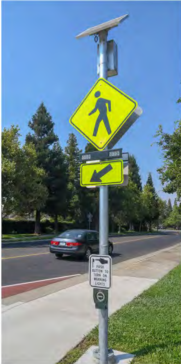
Figure 33 Rectangular Rapid Flashing Beacon
